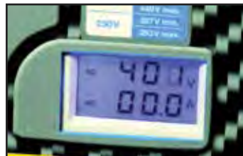
Volts and amps meter control display.
