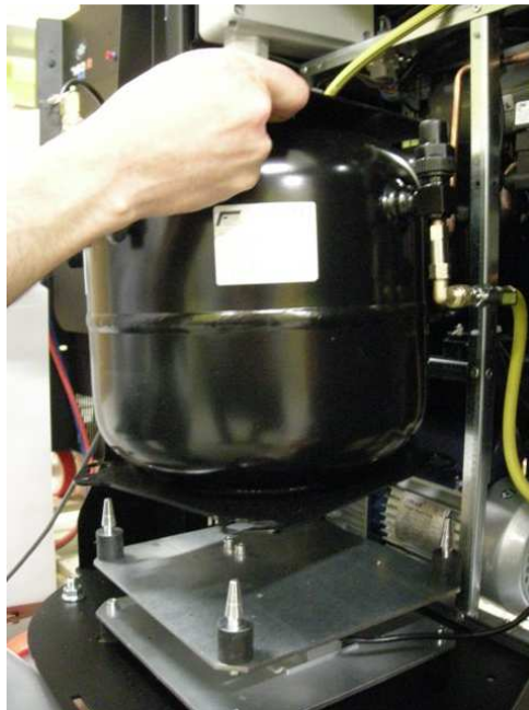
Image 4.25 – Lifting of the refrigerant tank during the calibration of the load cell in a Konfort 705R, 710R or 720R
