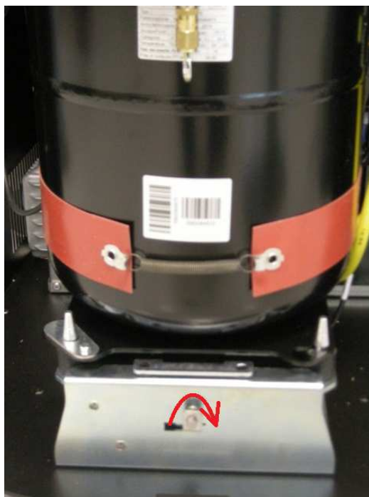
Image 4.46 – Refrigerant scale lock
