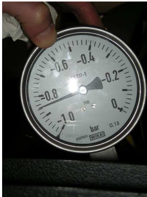
Image 7.20 – Depression level showing that the suction capability is appropriate
