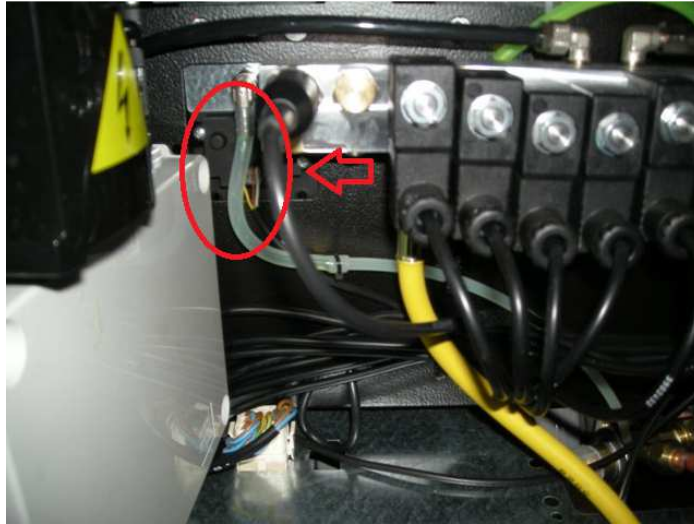
Image 7.40 – Silicone tube for the oil drain properly connected to its junction (See red circle)
