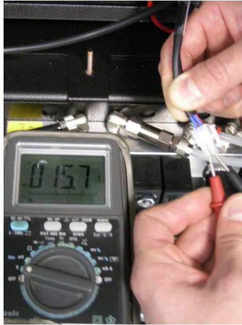
Image 7.7 - Between the two blue wires of the cable there must be an alternate voltage of about 15,5V
