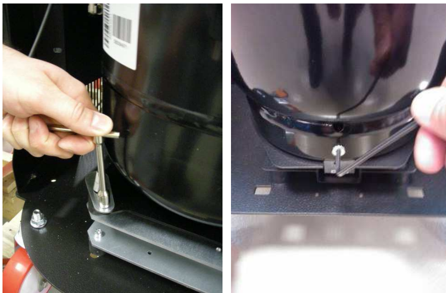
Image 4.22 – Removal of the bracket that blocks the tank to the structure of the scale
